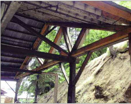
Here, the bottom chord of this truss is one continuous 80' Douglas fir timber.
